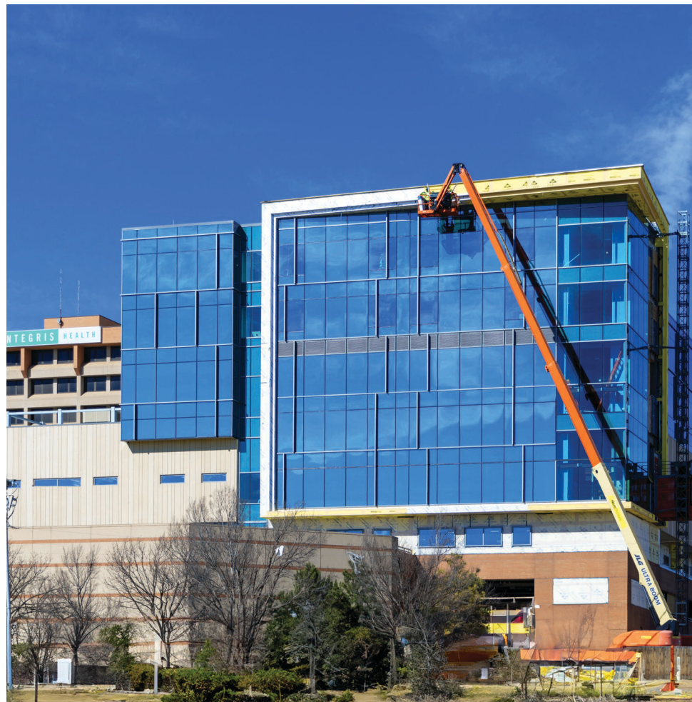
The new six-story Integrus Health Heart Hospital is expected to be completed in June. Photo provided.
